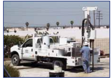
Many of our direct push rigs can be converted to hollow stem auger mode to eliminate the costly mobilization of a second rig.
