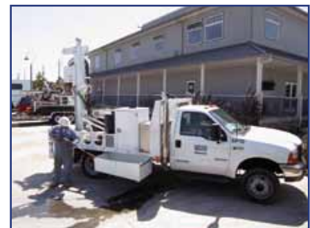
The truck mounted drill/probe rigs are equipped with on-board steam cleaners, grout mixing and pumping systems.
