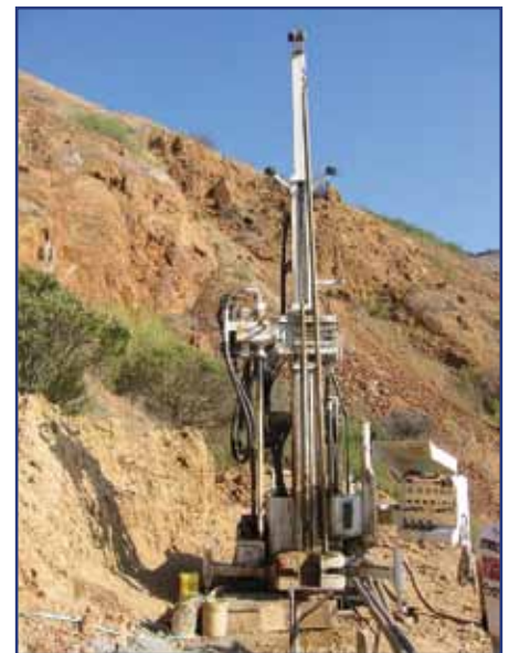
Slope Stability Investigation for Reclamation of Former Quarry Site - Track-mounted Fraste Mud Rotary Drill Rig
