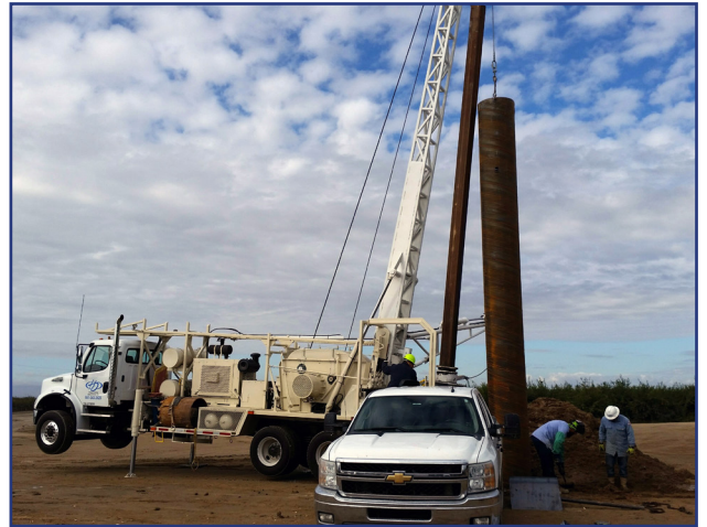
Above: Gregg Drilling's Fraste FS400 drill rig is an Italian made robust drill that can operate in direct mud rotary mode, or for deeper well installations, using reverse circulation.
