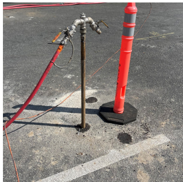
DPT INJECTION POINT
